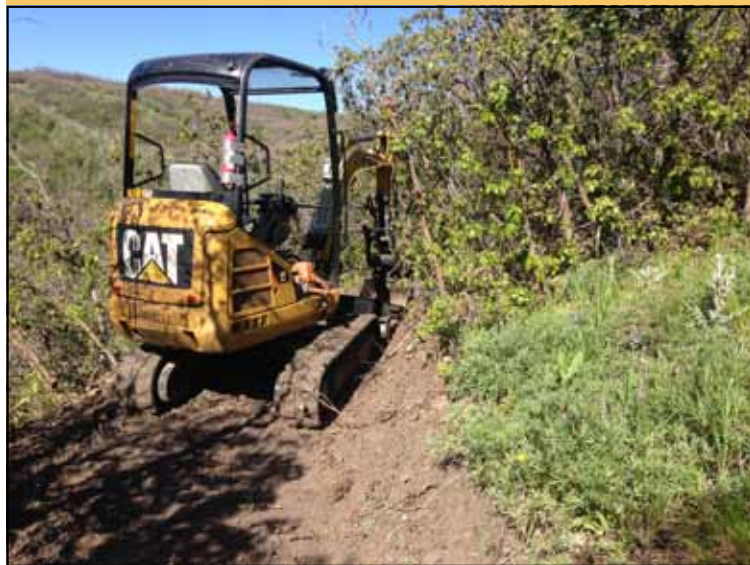
Mini excavators allow builders to make more trail with less hand labor. Photo by Donald West
