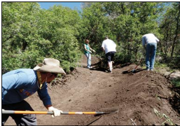
Above: Hand crews putting finishing touches on machine built berm. Right: Flow trails are fun to ride or run. Photos: Joey Klein/IMBA
